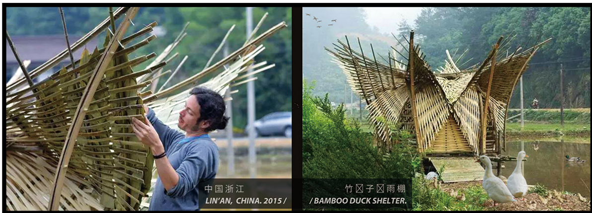
Figure 24: Bamboo duck shelter. Contribution to the ducks raising in rural Lin'an, Zhejiang, China. (April 2015).
